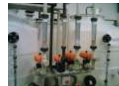
Close-up of typical pure piping array.
